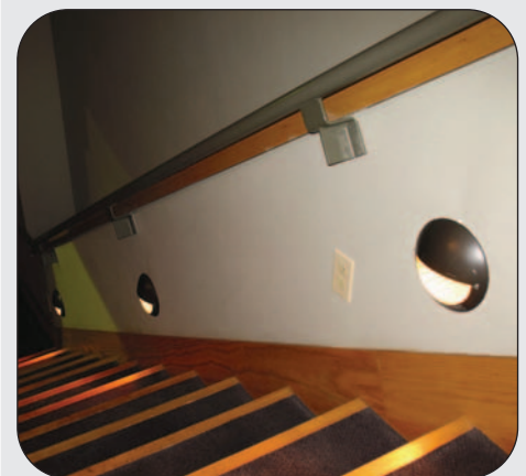
Clamshell fixtures are mounted to the walls illuminated the aisle and steps.
